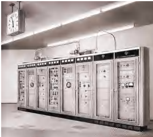
1963: VHF radio transmitter with 2 × 5 kW
