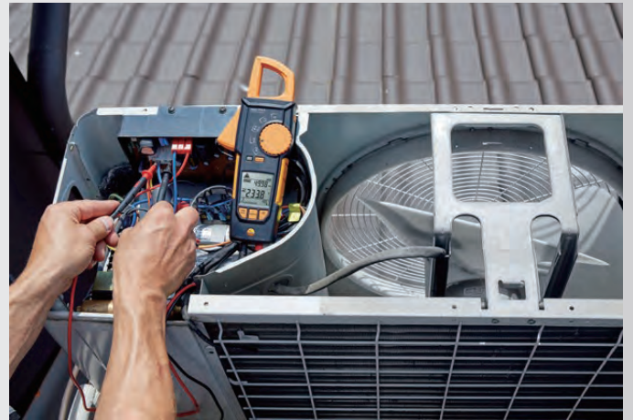
测量空调外机电压
