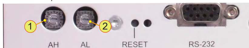
Fig. 32 Rotary switch AH -1- for the upper address range Rotary switch AL -2- for the lower address range
