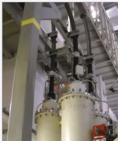
Terminations of a 380 kV buried cable system
