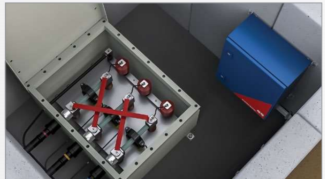
PD monitoring at the cross-bonded joints of a buried cable system
