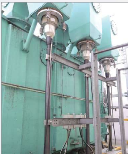
Terminations of a 230 kV short cable system
