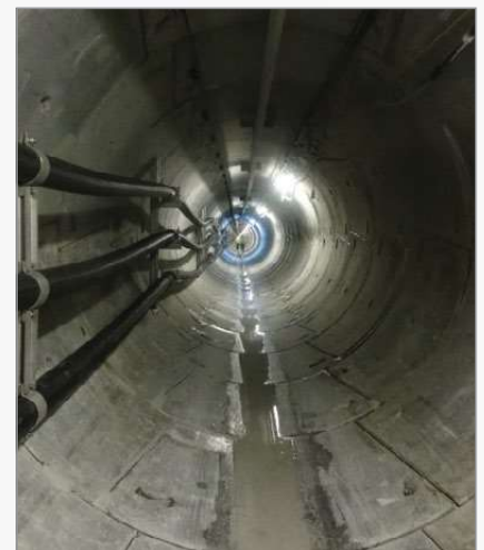
Joints of a 380 kV tunnel cable system
