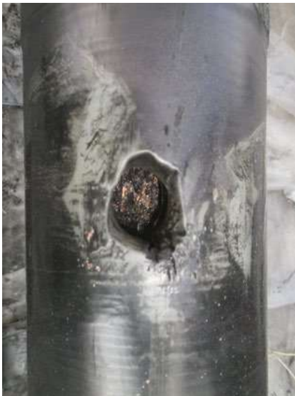
Insulation breakdown at a cable termination
